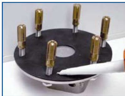
First thread the WAKO plugs onto the bolts (with neoprene washers), then apply sealant to the seal.
